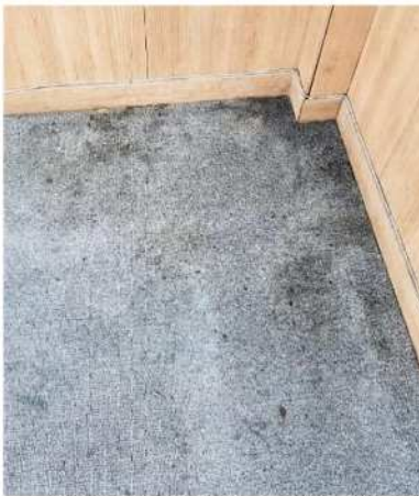
Accumulated stains & dirt
