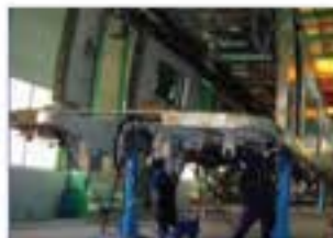
Electric Cable Connection
